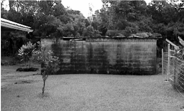
Hollow tile tanks have lost popularity mainly due to their price and tendency to leak.
